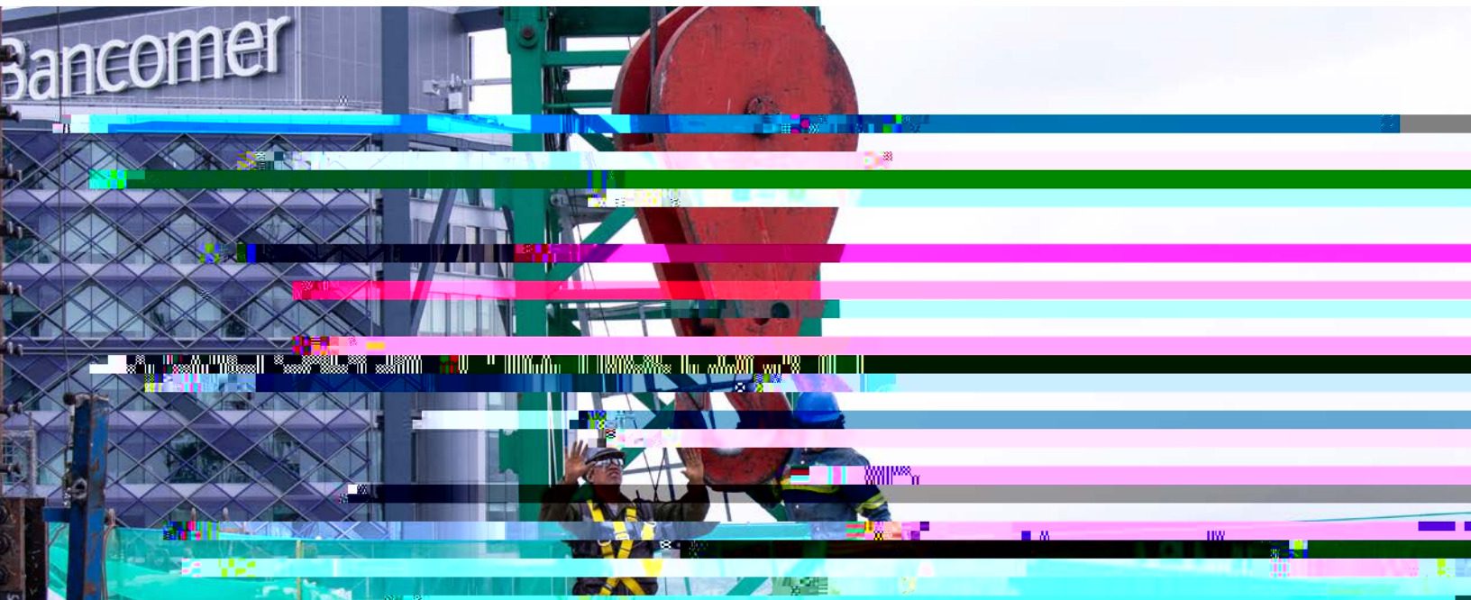
Construction workers are welding the steel frame for a skyscraper in Mexico City. Photo courtesy of: Luxbox/shutterstock.com
